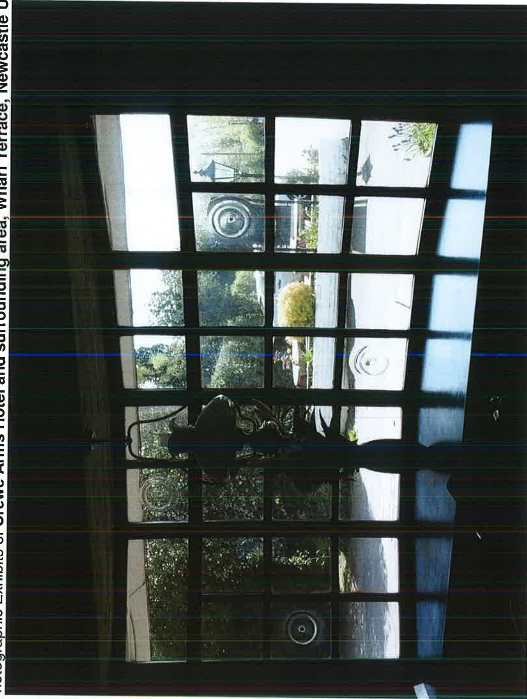
View from bar area to front of premises. Single glazed windows. Hedge line belongs to Ivydene
