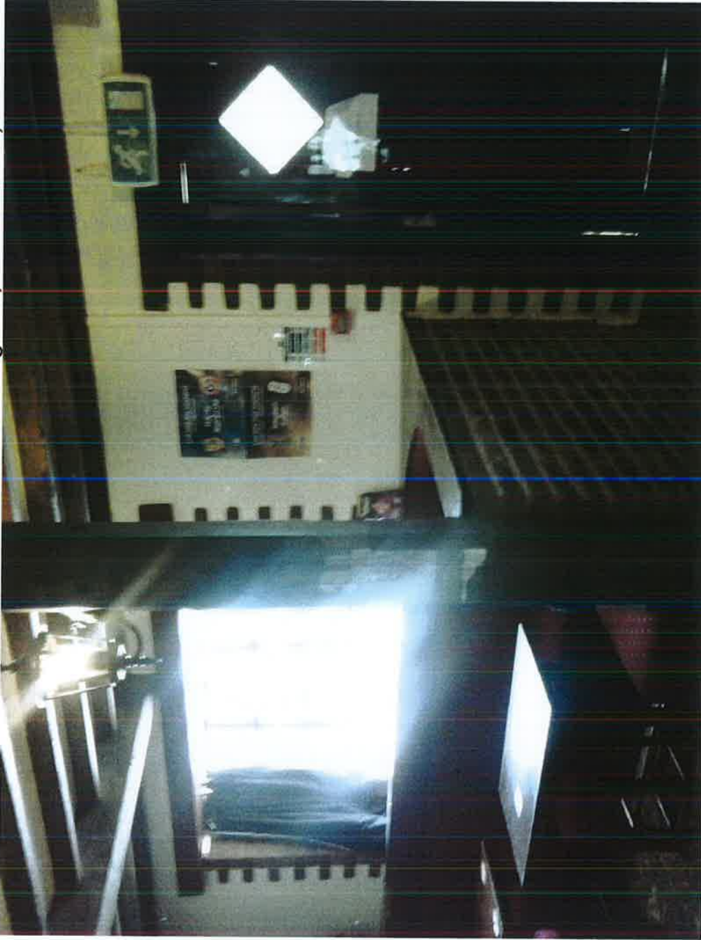
Main bar main entrance from car park at front. Door opens onto single glazed lobby
