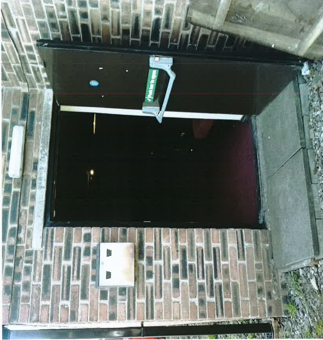
Fire door from function room – note cigarette bin on wall
