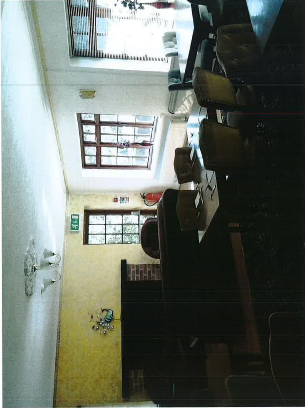
Function room opposite Ivydene Wharf Terrace. Single glazed windows and doors
