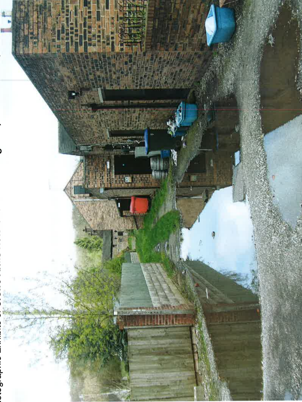
RTH 11 - View from Wharf Terrace (position 5) along the rear façade of the pub showing the function room fire door (right of centre), nearby farm (distant centre) and the boundary to nearby residential premises (left).
